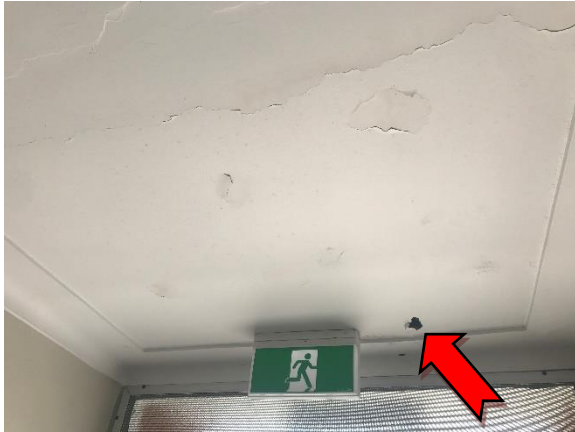
Photo 1. Interior, corridor, original ceiling above plasterboard ceiling – asbestos-containing fibre cement sheeting.
