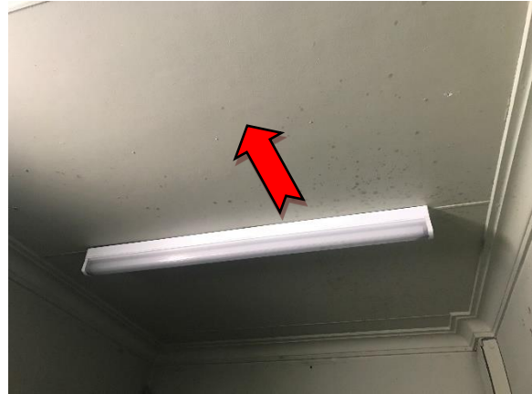
Photo 2. Interior, store 3, ceiling – asbestos-containing fibre cement sheeting.
