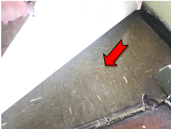
Photo 3. Interior, kitchen, floor coverings – asbestos-containing vinyl floor tiles.
