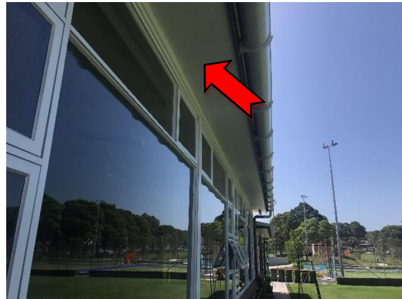
Photo 4. Exterior, throughout, eaves – suspected asbestos-containing fibre cement sheeting.
